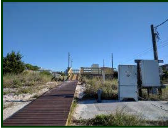
Improvements to Century Link Utility Area on Okaloosa Island: New Trex Walkway and New Service Platform (Stairs, Railings and Deck). Looks Good!
